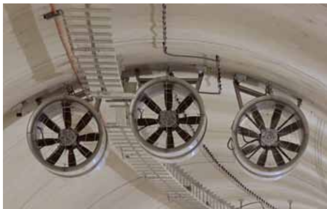
Example of a non-compensatable resource: smoke extraction ventilation system
