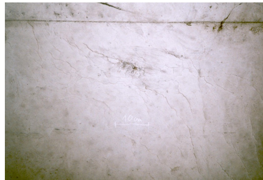
Figure 4: network of skin cracks
