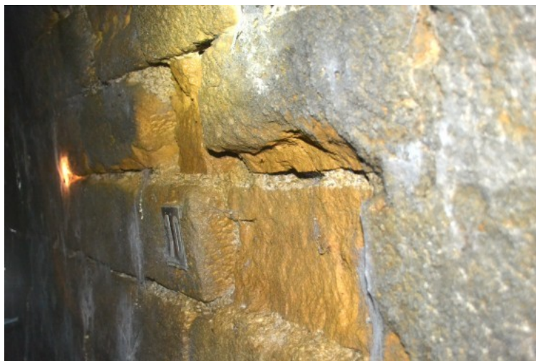
Figure 3: exfoliation and delamination of limestone masonry
