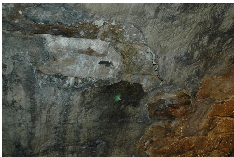
Figure 2: deteriorated waterproofing coating caused by water ingress (due to poor workmanship and effects of freezing)
