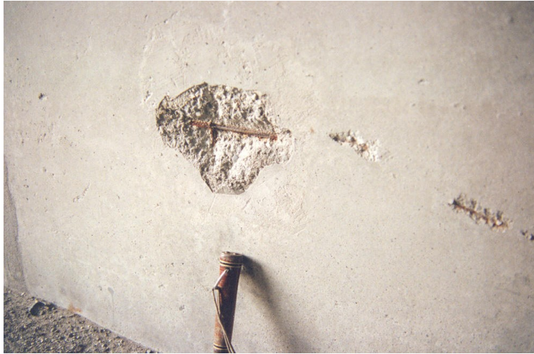
Figure 2: spalling in recent concrete
