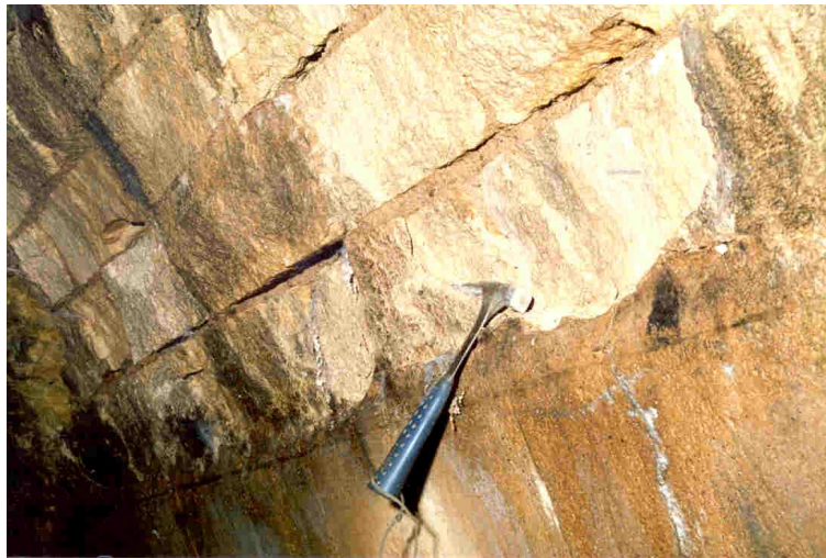
Figure 2: exfoliation of fragile, frost-susceptible oolitic limestone masonry
