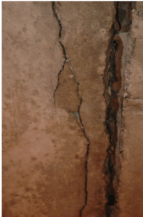
Figure 1: deterioration in an elastomer joint
