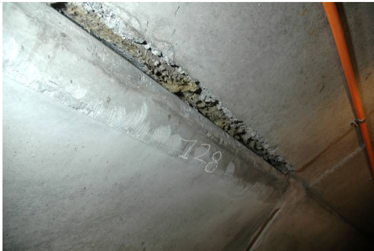
Figures 2a and 2b: chipping at the edges of slabs
