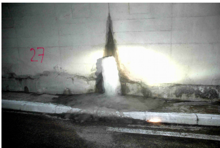
Figure 6: pack of ice coming from a joint and spreading onto the walkway
