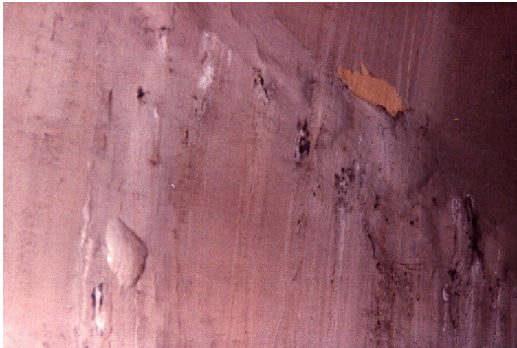
Figure 2: blisters in the resin membrane filled with pressurised water
