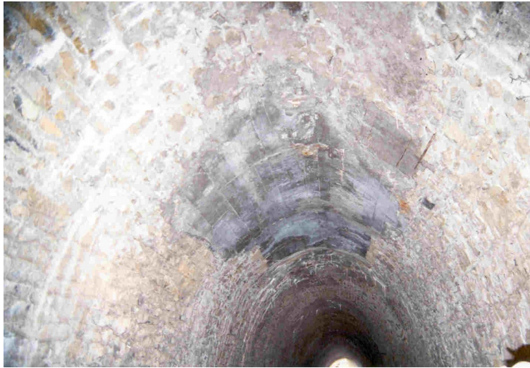
Figure 3: symmetrical squeezing in the crown (already partially repaired with non-reinforced cast concrete, the deformation is continuing, crushing the remaining crown stones and concrete)
