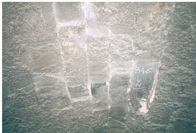
Figure 2: stone spalling at the crown (the parts that appear smooth are the scars left by fallen spalls up to 10 cm thick; note the almost total absence of mortar in the longitudinal direction, as well as a loosened spall still in place, held in place from the sides)
