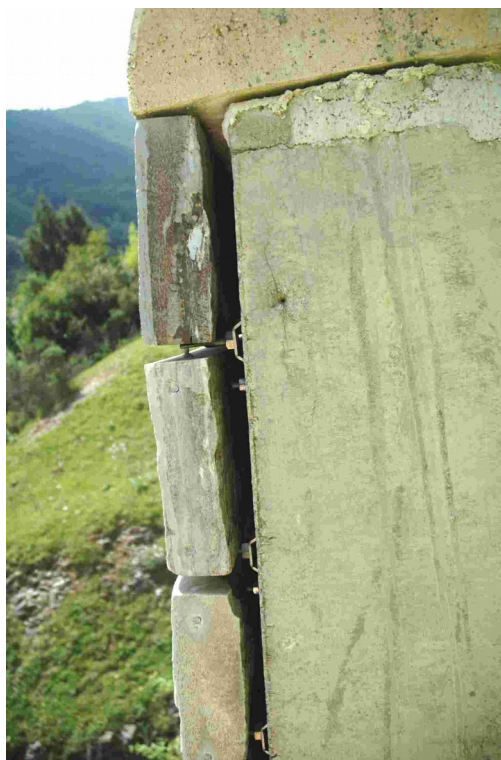
Figure 4: loosened panelling on a spandrel
