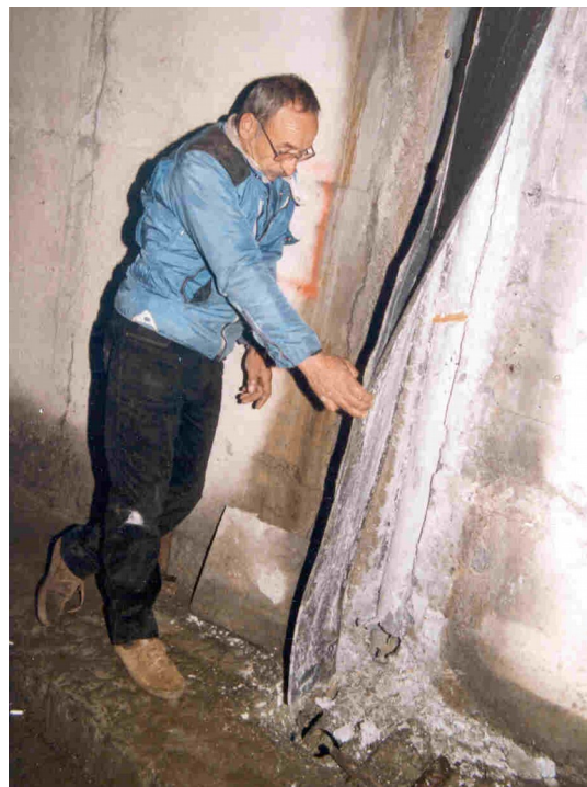
Figure 2: loosened sealing strip (the bottom of the collection system has been destroyed by freezing and is blocked)
