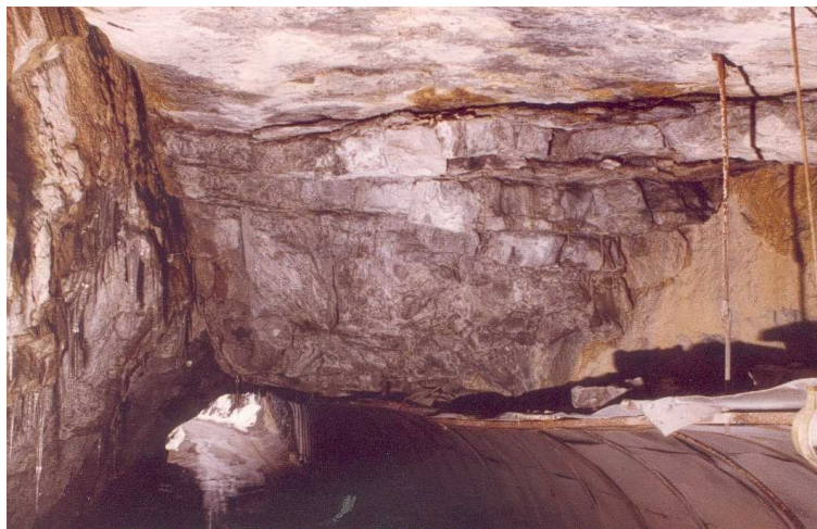
Figure 1: block that has fallen on metal sheeting, indicating weakening of the end of a limestone stratum (the presence of two damp vertical discontinuities at the sides constitutes a potentially hazardous long-term situation for the entire central part of the rock)
