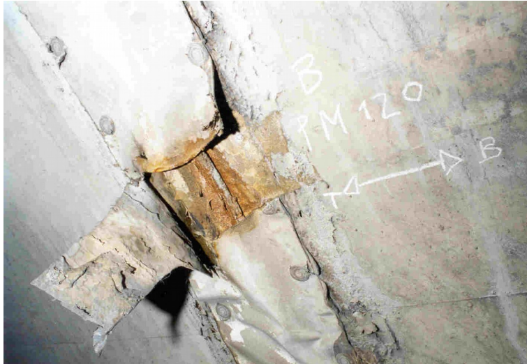
Figure 3: sealing strip and removable seal (here PRT seal and Hypalon sealing strip) destroyed by friction from heavy goods vehicles
