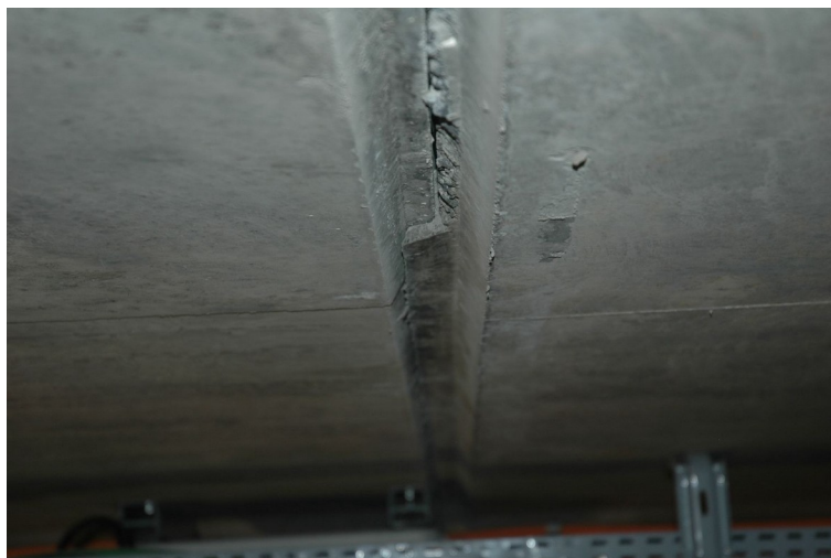
Figure 4: deterioration of a dry joint [movement between rings or concrete breakage during form removal]
