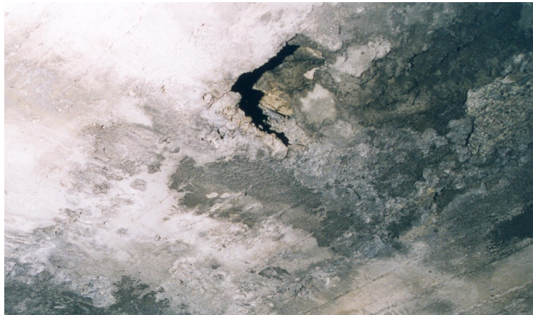
Figure 2: void dating back to construction, on the extrados of highly deteriorated concrete [the hollow-sounding lining is unstable around the opening]
