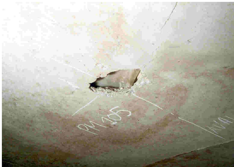
Figure 1: fold in membrane (localized hollow-sounding area)
