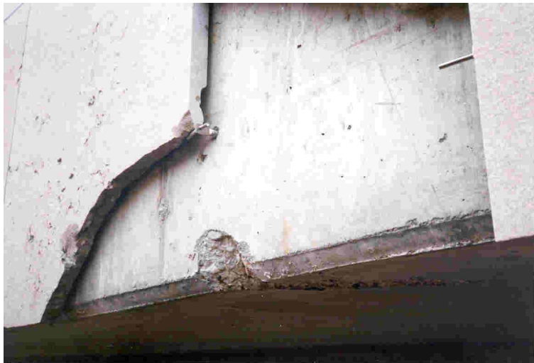
Figure 3: fallen cladding due to impact from a heavy goods vehicle
