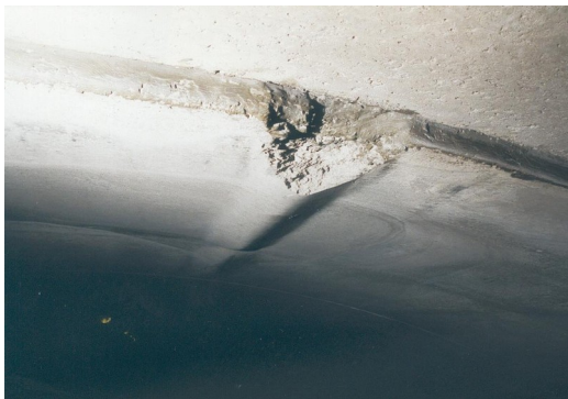
Figure 1: localized formwork deformation
