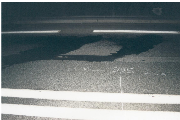
Figure 2: water rising through asphalt
