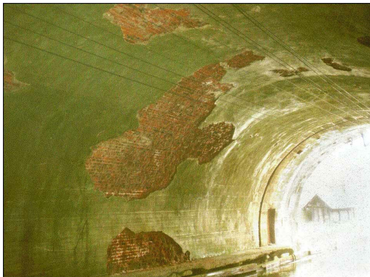
Figure 2: fallen coating (brick arch in a canal tunnel)
