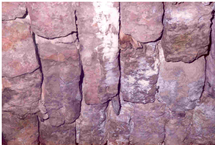
Figure 2: joint disintegration, typical of a lack of maintenance (wood dowels were probably used to secure stones or stop local water ingress; the stones, although of good quality, have almost come loose)
