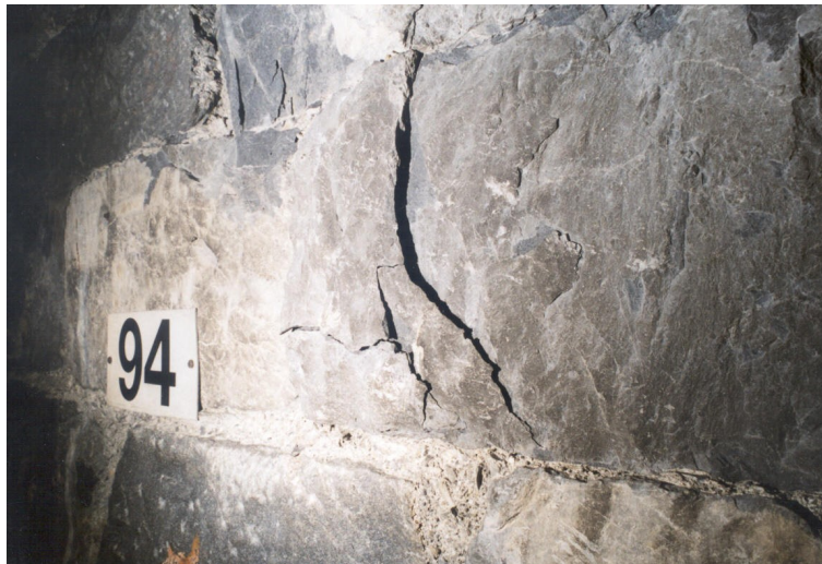
Figure 3: stone spalling on the side wall (the spall has broken away 15 mm from the wall and cannot be detached by hand; the upper and lower stones are in direct contact, as there is no mortar)
