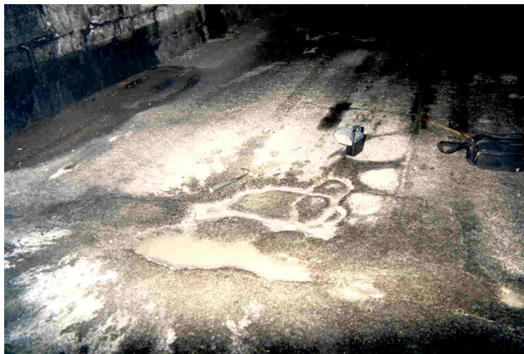
Figure 1: crazing and potholes [foundation saturated with water, with areas dissolved under the effect of pumping resulting from the passage of vehicles]
