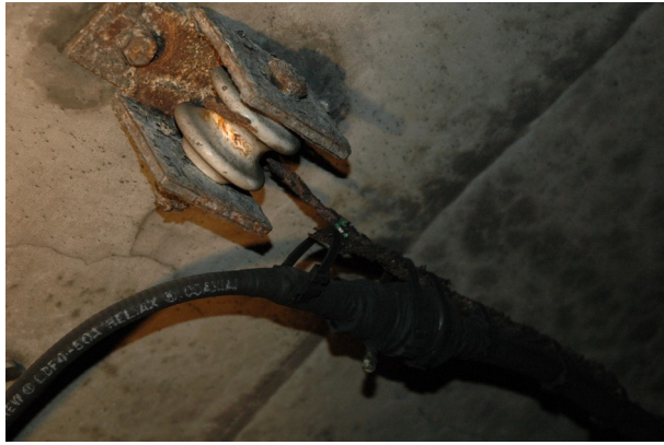
Figure 2c: broken plastic power cable fixture in the roof section
