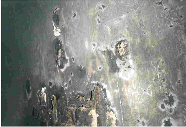
Figure 1: deterioration of a resin membrane installed on masonry
