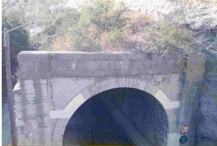
Figure 1: cracking and lateral tilting of a spandrel, untreated rockfall canopy
