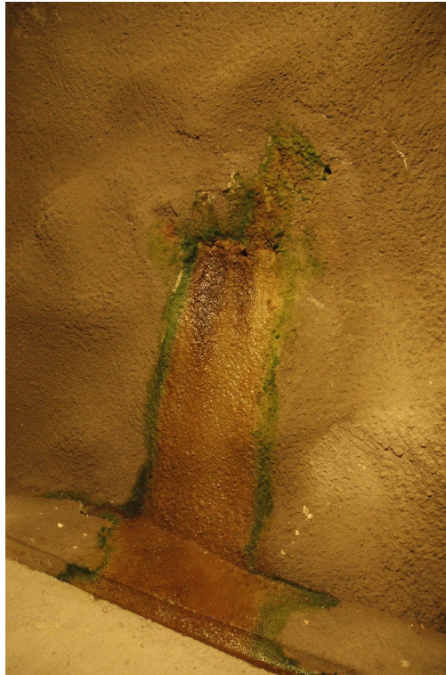
Figure 1: water ingress on a sprayed concrete lining
