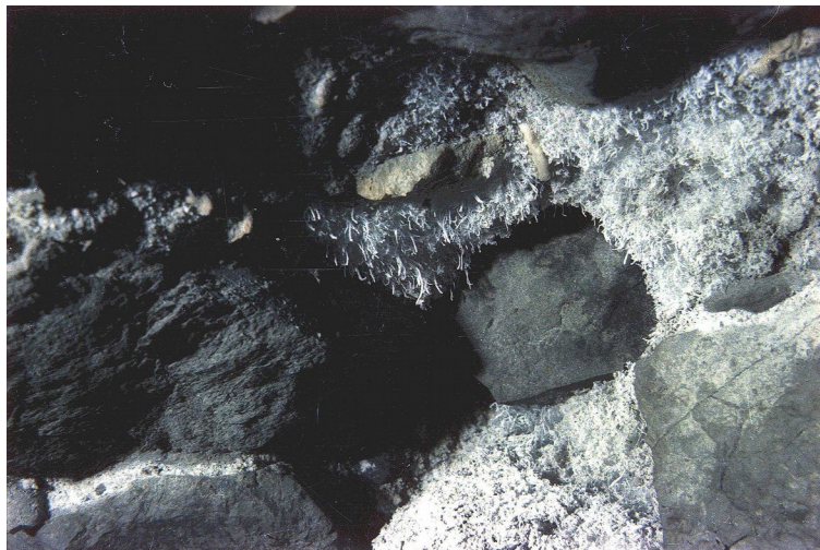
Figure 1: efflorescence on old lime-based mortar
