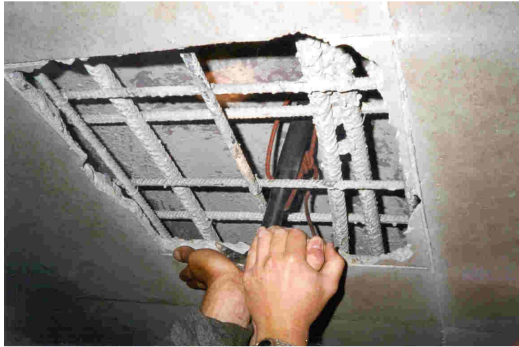
Figure 1: investigation window opened in a very hollow-sounding area [extrados void of 27 cm due to a concreting defect]
