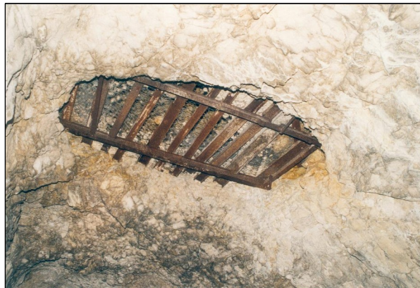
Figure 1: metal bars used as protection against falling, poorly consolidated materials from a karst
