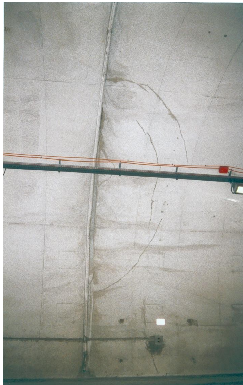
Figure 1: nested curved cracks in the haunch (the bottom of the photo corresponds to the walkway; concreting was carried out from right to left)
