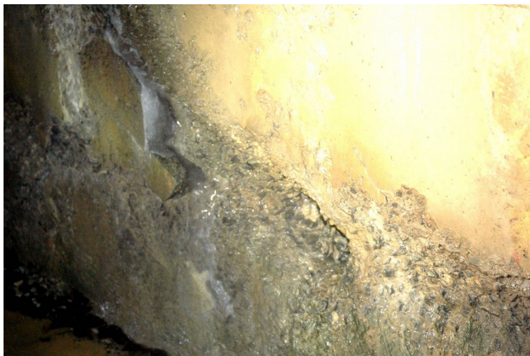
Figure 5: spalling of concrete due to freezing, at the bottom of the side walls
