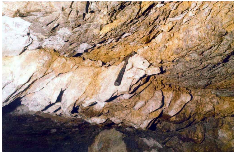
Figure 1: fractured mass separated from the surrounding rock by a clayey joint or "unstable rock bridge" (scaling is possible as an initial measure)
