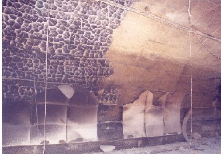
Figure 1: crazed concrete [thermal limit clearly shown where soot is deposited on the crazing], at a distance of 120 m from the heavy goods vehicle that caused the fire in the Mont-Blanc tunnel [no other vehicle involved]
