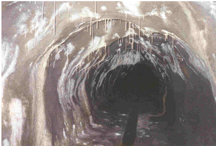
Figure 2: stalactites and white calcite flowstones on sprayed concrete (dissolution of the lime in the cement due to water percolating from the ground)
