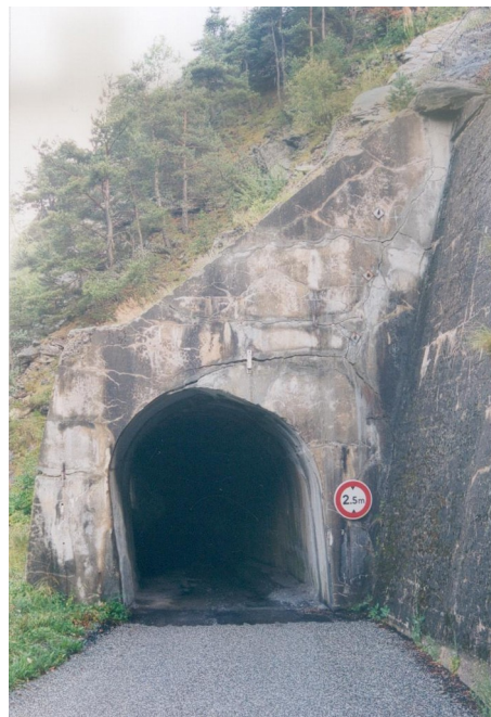
Figure 2: portal deformed by slope instability
