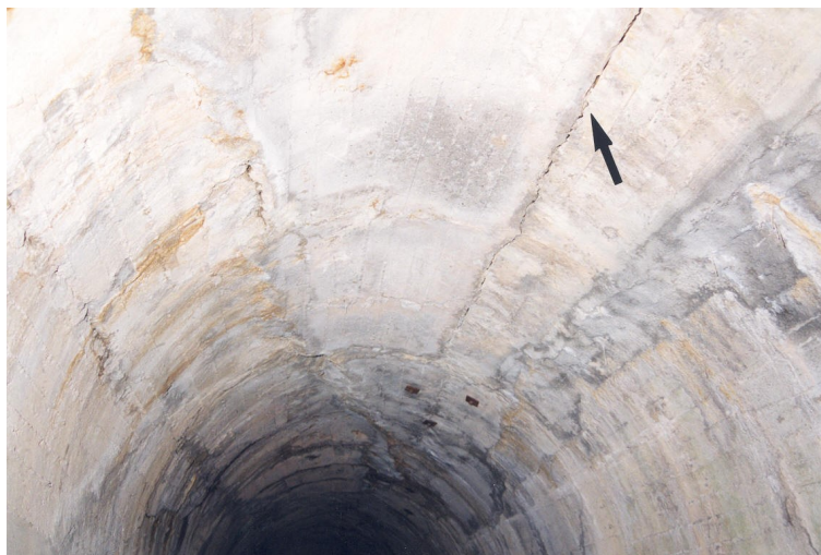
Figure 2: horizontal crack in cast concrete related to deformation of the lining under the thrust of the surrounding ground (the crack forms along the construction joint)
