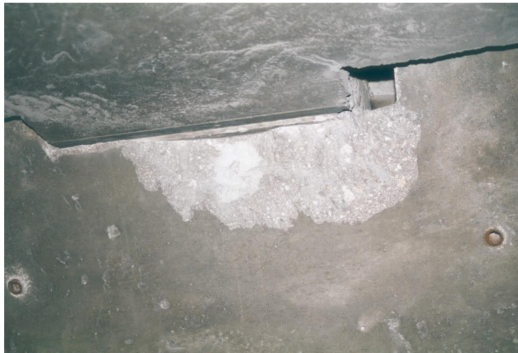
Figure 1: spall fallen from beneath a trench
