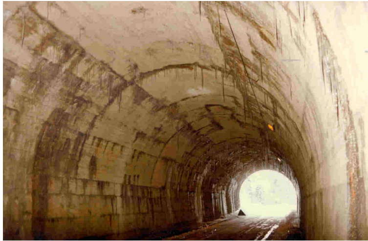
Figure 1: gravel pockets on a concrete lining from 1936 [each layer of concrete is highlighted by an alignment of permeable and perfectly horizontal gravel pockets due to poor concreting]
