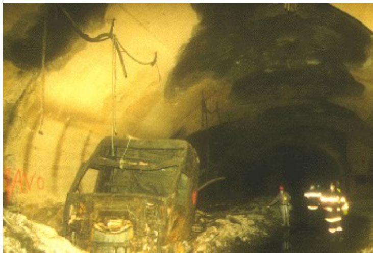
Figure 2: craters 30 to 60 cm deep created in the arch by the fire next to the heavy goods vehicle that caused the fire [Mont-Blanc tunnel]
