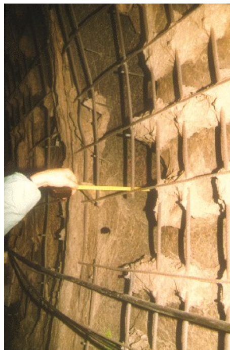
Figure 3: deep spalling revealing the intrados reinforcements, following the ten-hour fire in the Channel Tunnel in 1996, involving a heavy goods shuttle. In the most affected area, at the heart of the fire in this tunnel, (formed of prefabricated reinforced concrete segments), the damage locally affected the tamping mortar.
