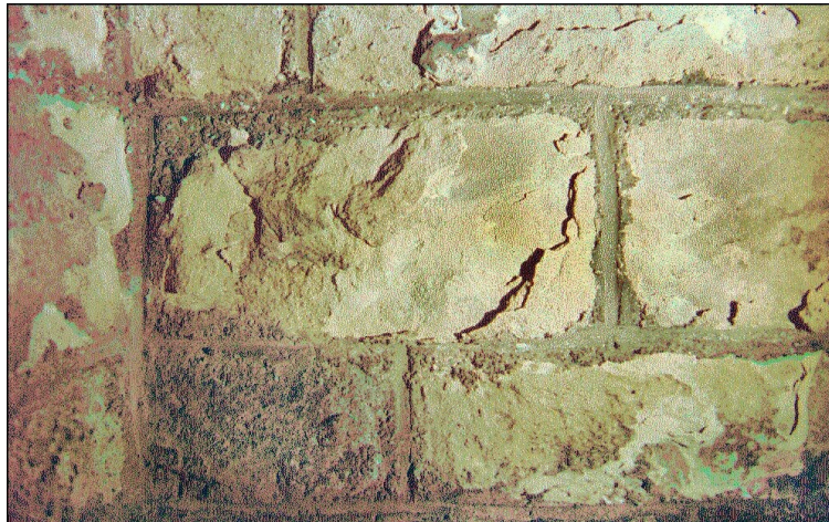
Figure 1: flaked stone (the sandstone masonry has been repointed some time ago using a compact and cement-rich mortar that has probably accelerated or even initiated the flaking process by enabling water to enter the stone)
