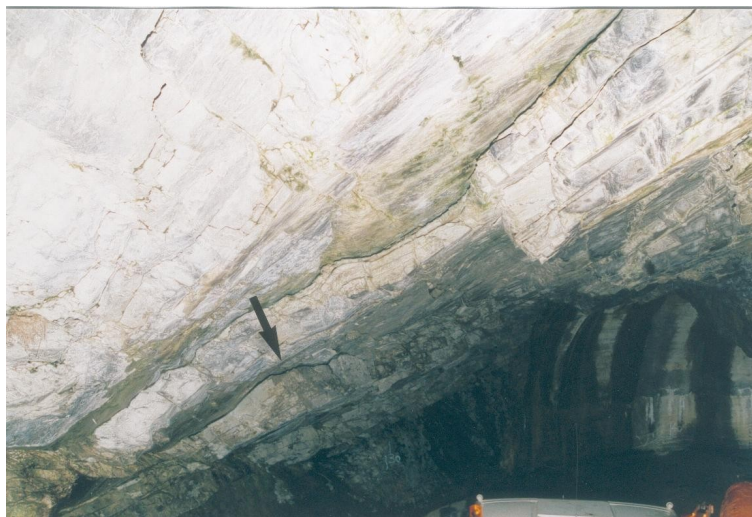
Figure 2: loosened plates at a 45° angle in the tunnel haunch
