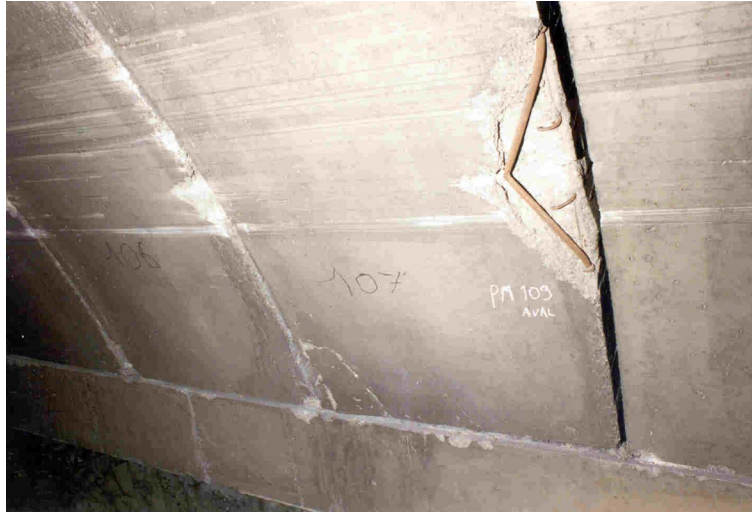
Figure 1: chipped thin prefabricated element following an impact (traces of friction)
