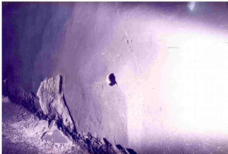
Figure 1: cracked and loosened coating on old concrete
