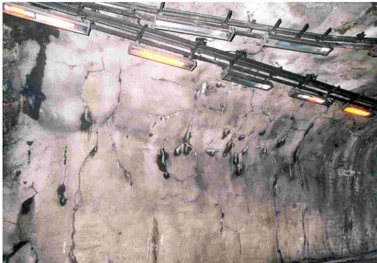
Figure 2: sprayed concrete crazing over damp rock (shrinkage of non-reinforced concrete)
