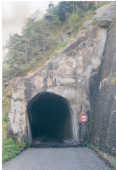
Figure 1: portal deformed by slope instability
