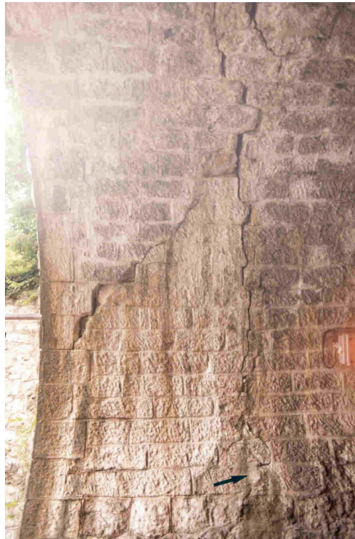
Figure 1: vertical crack combined with a diagonal crack
