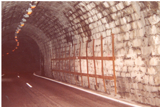
Figure 1: a bulging side wall, strengthened by anchors and tie rib
