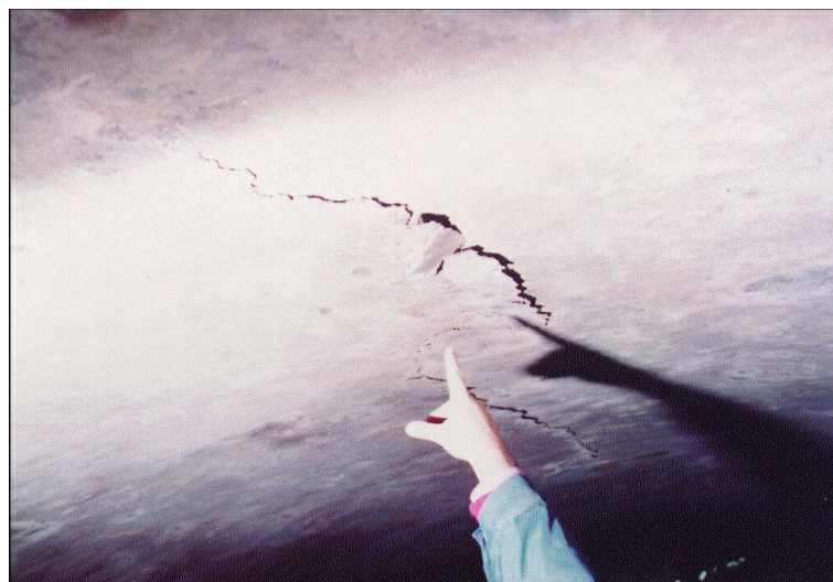
Figure 2: start of concrete shearing in the crown (the shear crack is shown clearly here; the edge is fragile)
