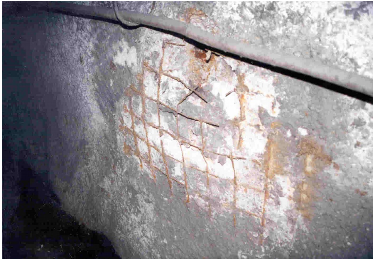
Figure 1: insufficient covering of the welded mesh (poor workmanship)
