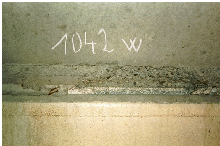
Figure 2: chipping at the bottom of a ventilation slab support that probably occurred during form removal; on the left, a spall remains that has not yet fallen
