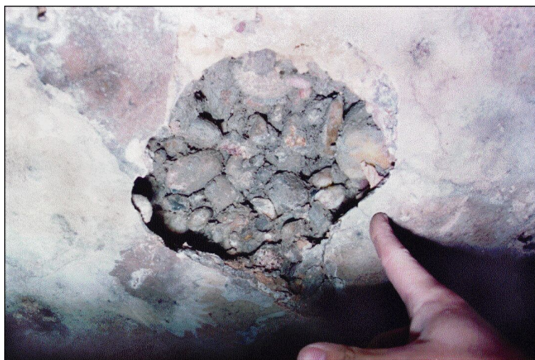
Figure 2: gravel pocket initially hidden by a film of laitance [its spread can only be mapped using hammer tapping]
