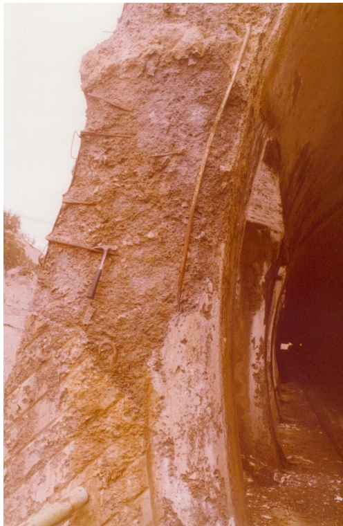
Figure 4: frozen reinforced concrete side wall
