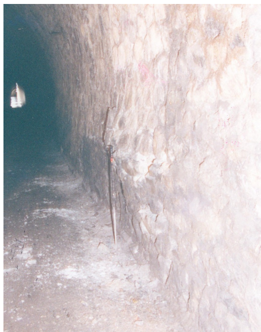
Figure 2: bulging nearing the stage of permanent damage (significantly deteriorated masonry)
