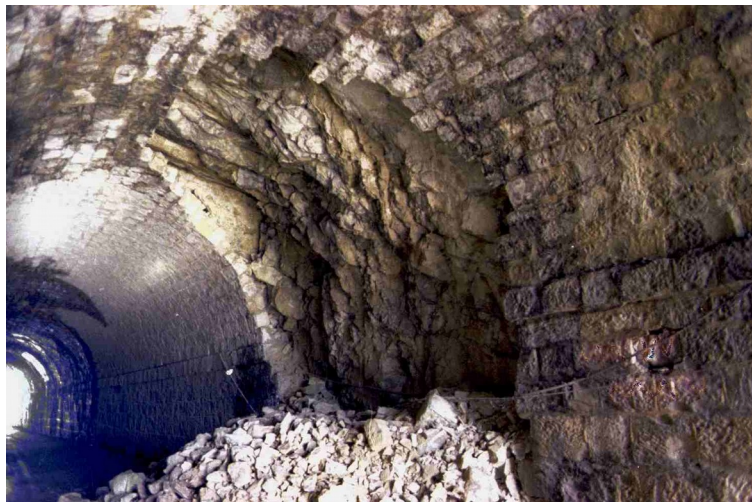
Figure 1: half the arch has fallen due to crushing of the side wall, consisting of very deeply delaminated, weak stones (this permanent damage was preceded by bulging of the side wall, which was not strengthened in time; the ground was not the cause of the deterioration)
