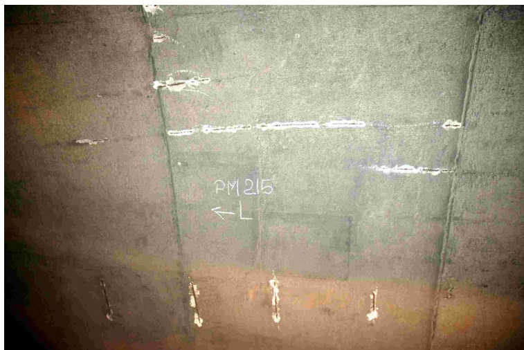
Figure 4: concrete spalling due to corrosion and thin covering of reinforcements
