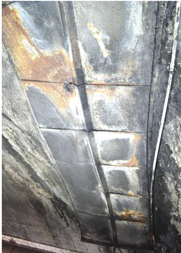
Figure 4: corroded and leaking zinc-plated steel intrados drain
