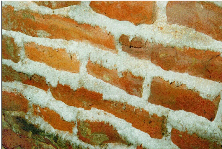
Figure 2: efflorescence on old lime-based mortar
