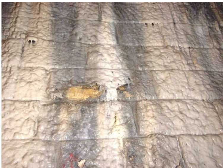
Figure 6: stone masonry encrusted with calcite concretions
