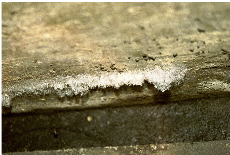
Figure 3: efflorescence at ground level on concrete from 1976
