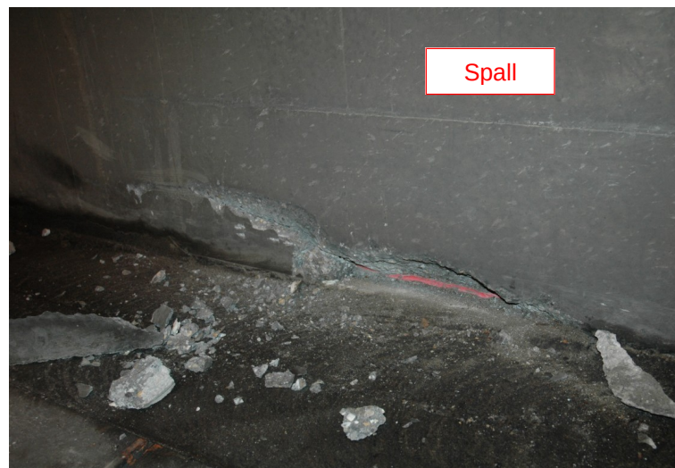
Figure 2: concrete spalling along the joint between the walkway and the side wall
