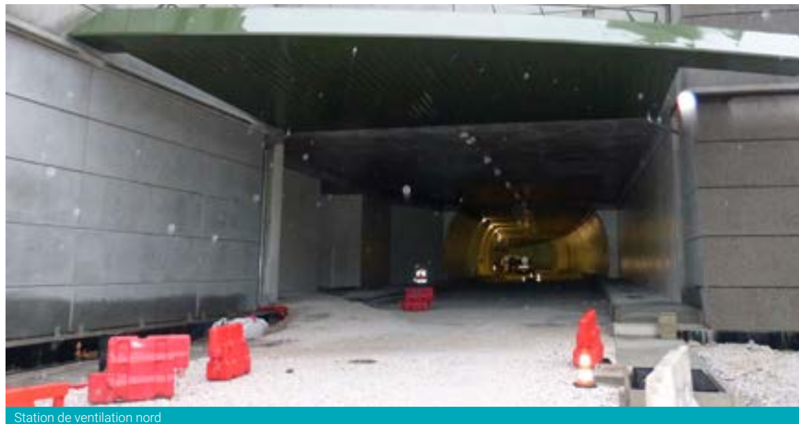
Station de ventilation nord
