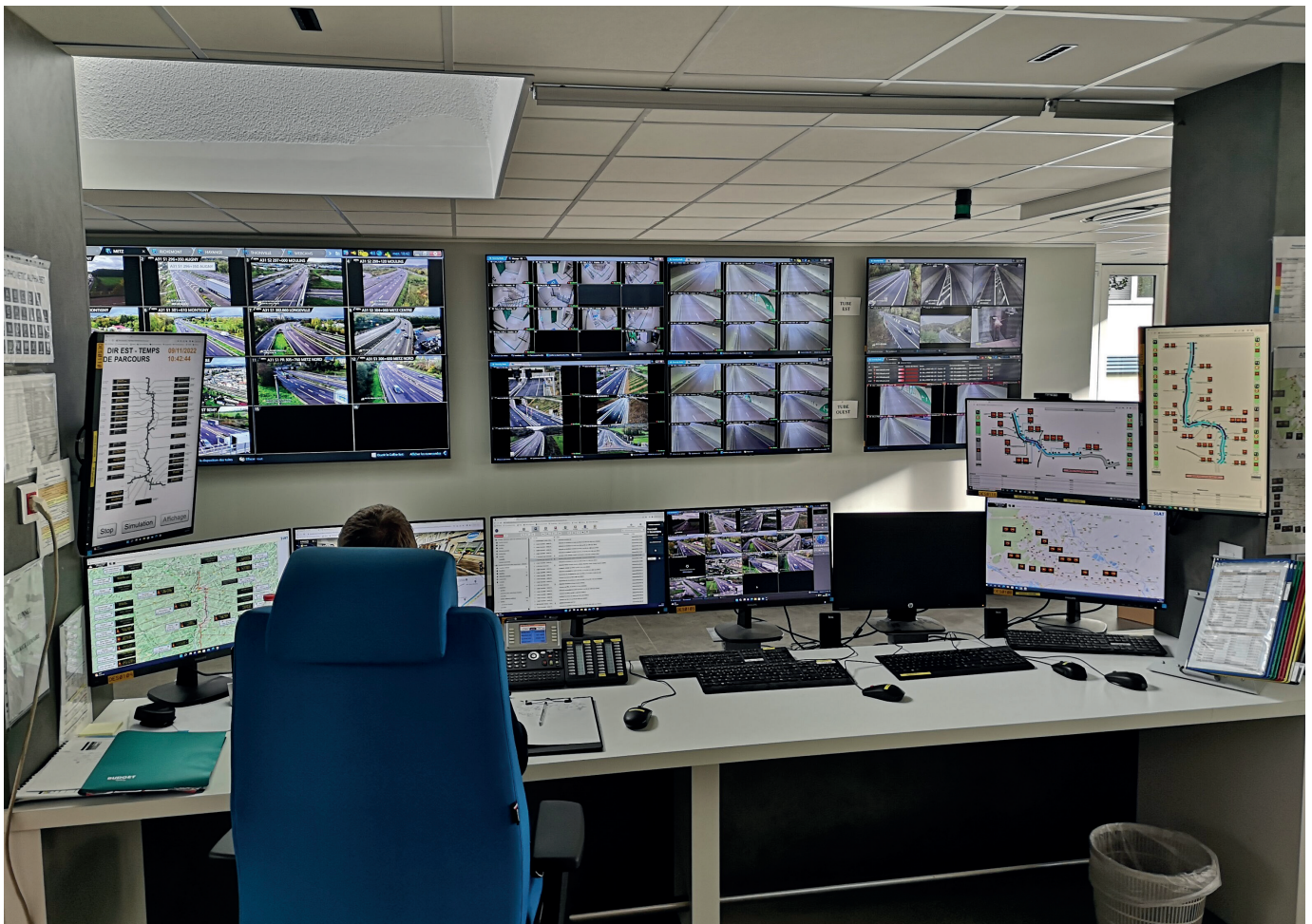
Figure 1: Video wall at the Control and Command Centre of the Traffic Management and Safety Centre in Moulin-les-Metz
