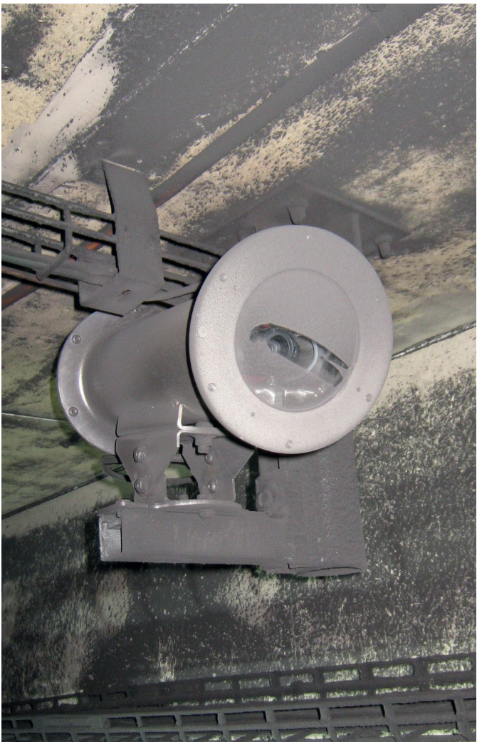
Figure 15: Dirt on the housing window of an AID camera
