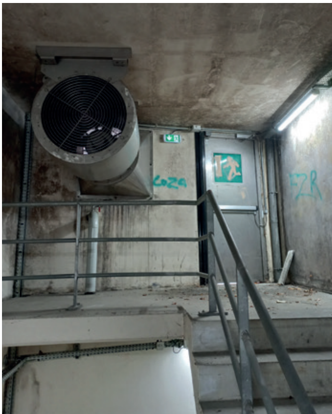
Lilas cover – Emergency exit (© City of Paris)
