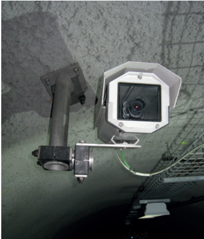
Montets Tunnel – CCTV camera (© CETU)
