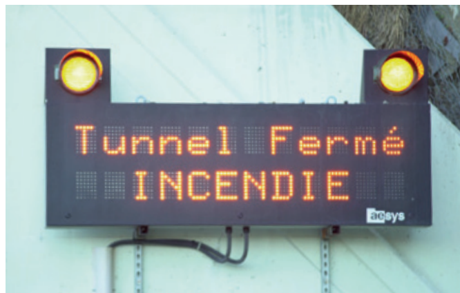
Baza Tunnel – VMS at the tunnel entrance during a safety exercise (© DIRMC)
