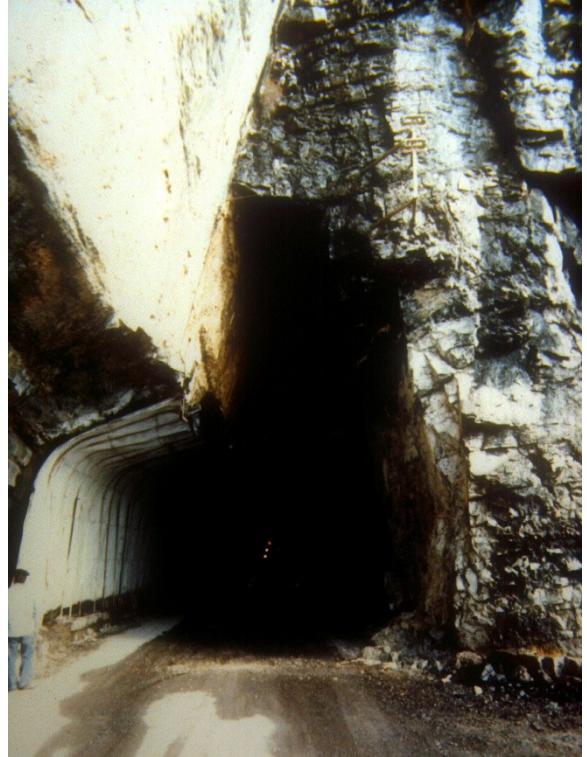
Figure 14b: condition three years later
