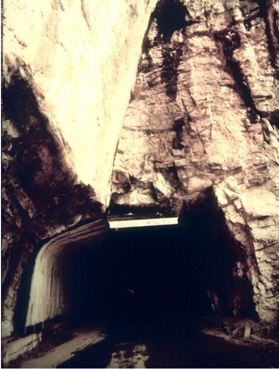
Figure 14a: condition at the time of the first inspection
