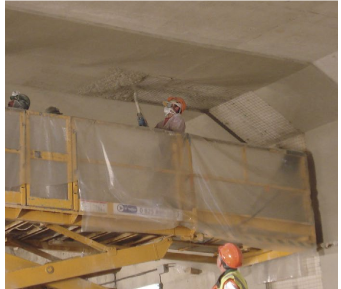
Sprayed type fire protection
