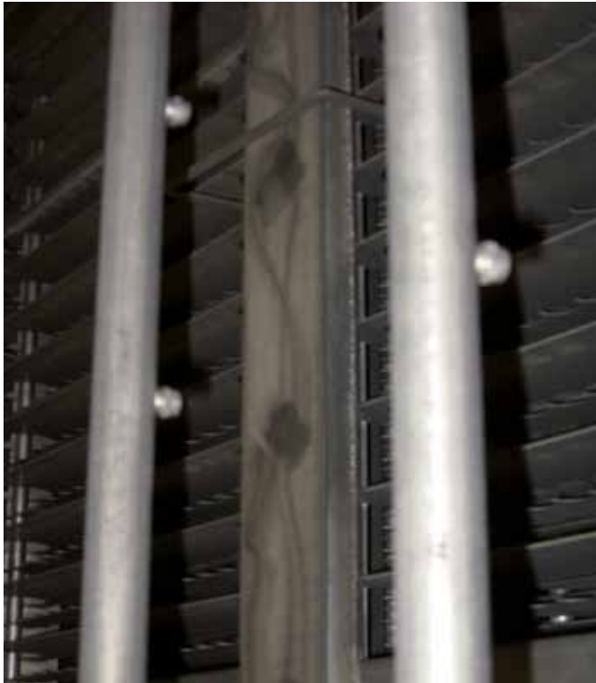
Illustration 25: rinsing nozzles on an ionisation device (CTA)
