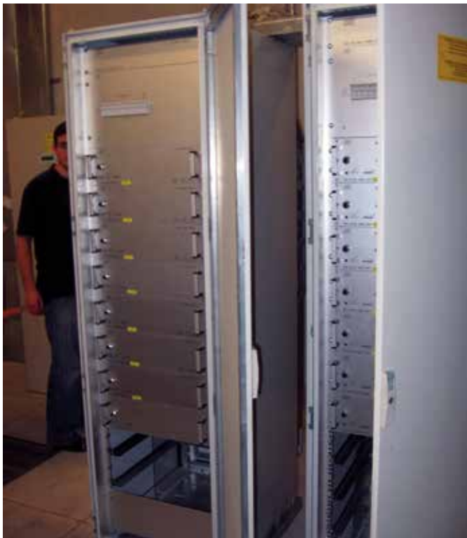
Illustration 34: cabinets containing the basic conversion units for the ionisation current (CTA)
