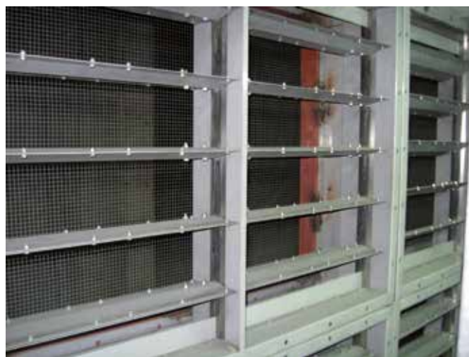
Illustration 20: air treatment circuit intake – close-up of the dampers and pre-filtration meshes (Aigner)
