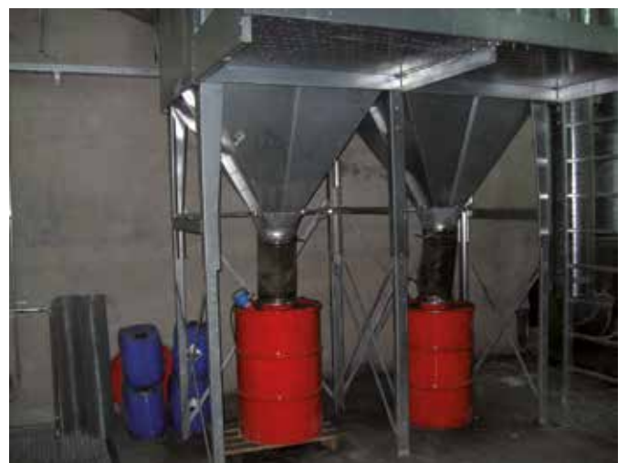
Illustration 37: collection of treatment residues at the end of the system for rinsing filters (Aigner)
