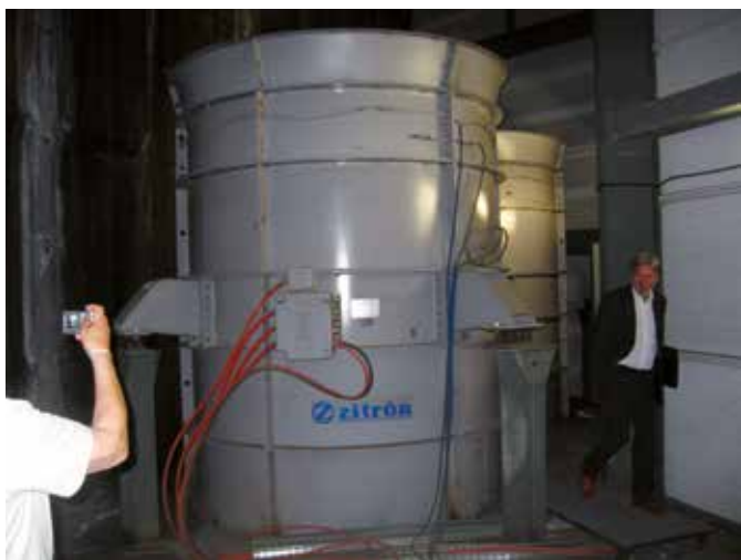
Illustration 18: Extraction fans used for both smoke extraction and air treatment, in vertical position (By-Pass Sur tunnel) – unit characteristics: 116 m 3 /s, 560 kW
