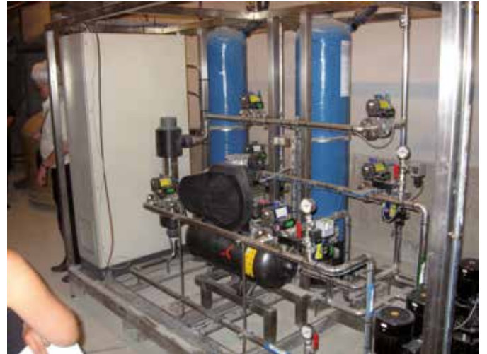
Illustration 35: installation of the system for treating water used to wash filters (CTA)
