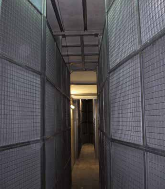
Illustration 29: DeNOx system – air circulates between the panels seen in the photo, from the back to front – the curved shape increases the panels' surface area (W-shaped profile when seen from above) and therefore, those of the contact surfaces between air and the activated carbon, thus enhancing system performance
