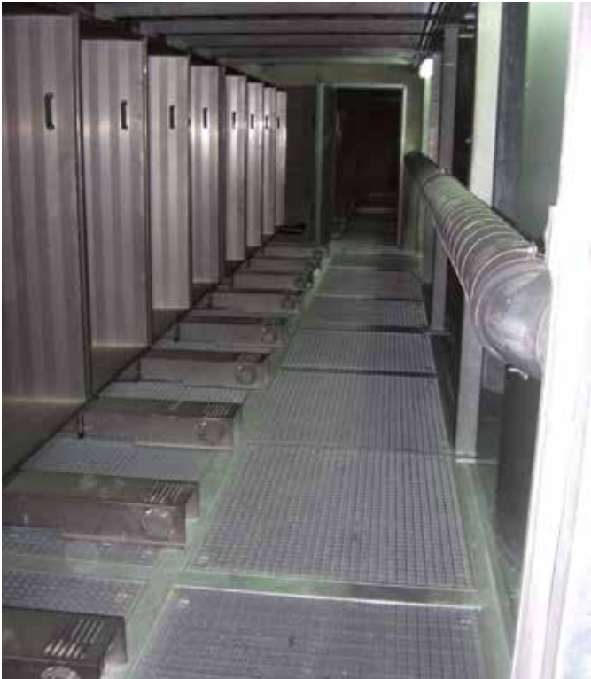
Illustration 23: on the left, cabinets containing the electrostatic filters and, on the right, deNO x system (air circulates from left to right)
