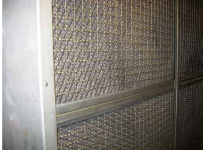
Illustration 31: DeNOx system – close-up of the panels housing the activated carbon pellets
