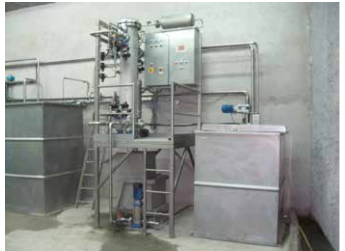
Illustration 36: installation of the system for treating water used to wash filters (Filtrontec)
