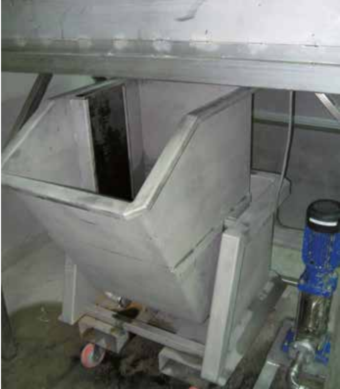
Illustration 38: collection point for treatment residues at the end of the system for treating water used to wash filters (Filtrontec)
