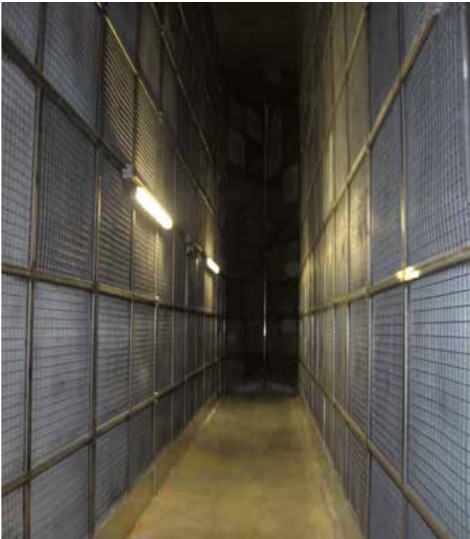
Illustration 30: DeNOx system – air circulates between the panels seen in the photo, a length of several metres is required to ensure a large enough contact surface area
