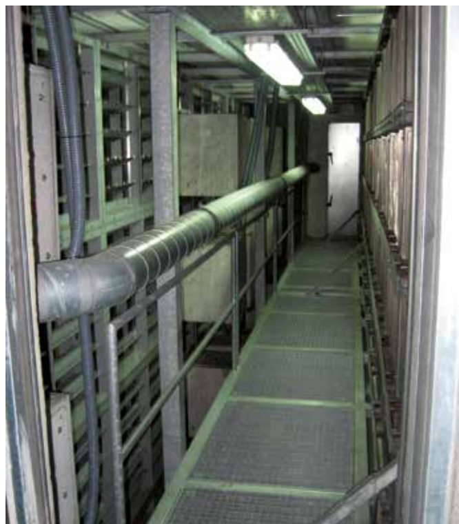
Illustration 19: air treatment circuit intake (air circulates from left to right) – on the left – opening/closing dampers for the treatment circuit, on the right, the ionising devices
