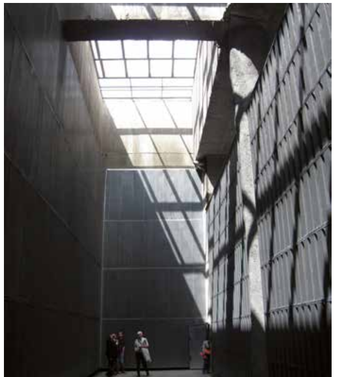
Illustration 32: end of the treatment system (air flows in on the right, fills the plenum then flows out through the opening in the ceiling) – on the right – the acoustic panels demonstrate the size of the aerualics section required to limit flow speeds through the system – at top right, in shadow, the opening that forms the end of the sheathing parallel to the treatment circuit making it possible to short-circuit the treatment system in the event of fire
