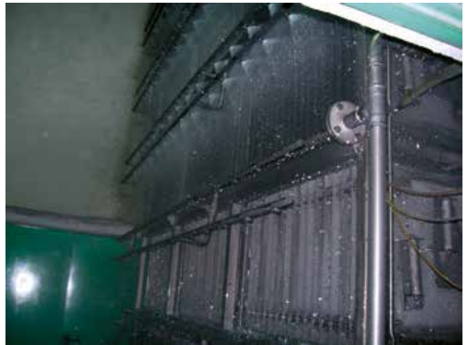
Illustration 28: filters being washed under high-pressure water jets (Filtrontec)
