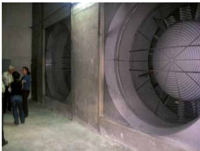
Illustration 17: Extraction fans used for both smoke extraction and air treatment, in horizontal position (cut-and-covered tunnel) – unit characteristics 203 m 3 /s, 630 kW
