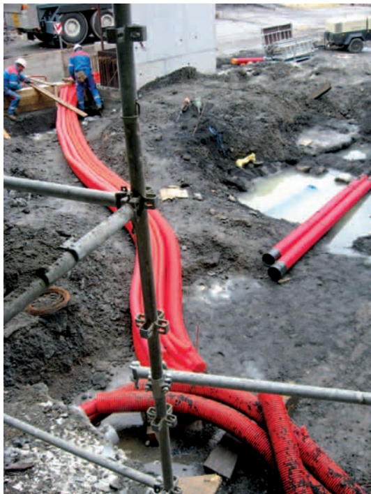
Photo 13: cabling tubes in the Lioran tunnel (source: CETU)
