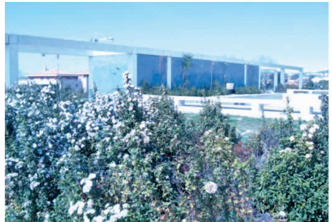
Photo 24: ventilation plant for the Montolivet cut-and-cover section on the L2 east of Marseille (source: CETU)
