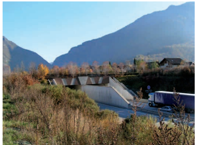
Photo 6: absorbing acoustic facings on the A43 in the Maurienne valley (source: CETE Lyon)
