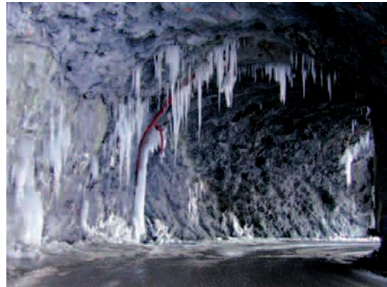
Photo 19: water inflow in a tunnel during winter (source : CETU)
