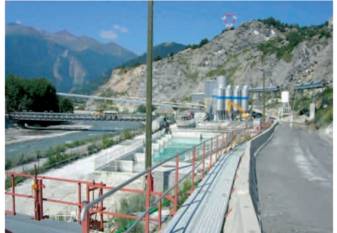
Photo 20: treatment basin at the Modane decline as part of the works on the Lyon Turin rail link (source: CETU)
