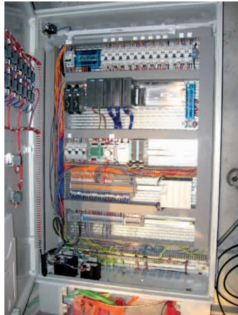
Photo 12: electrical cabinet in Lioran tunnel (source: CETU)
