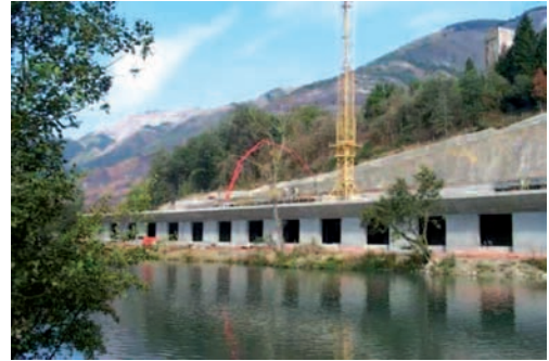
Photo 3: external view of an openwork cut-and-cover section along the Gave de Pau (source: http://www.midi-pyrenees.equipement.gouv.fr )
